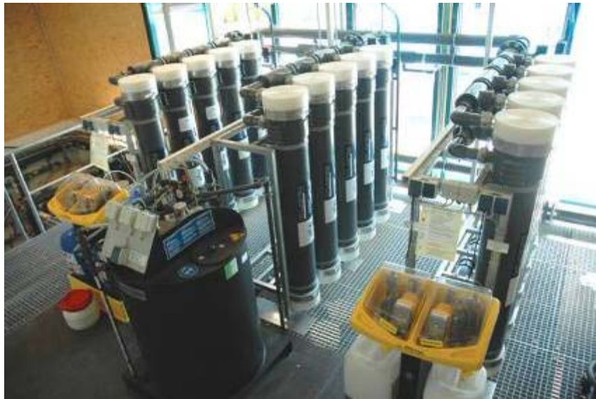
Ruhstorf (pool) - circulation water approx. 240 m 3 /h
